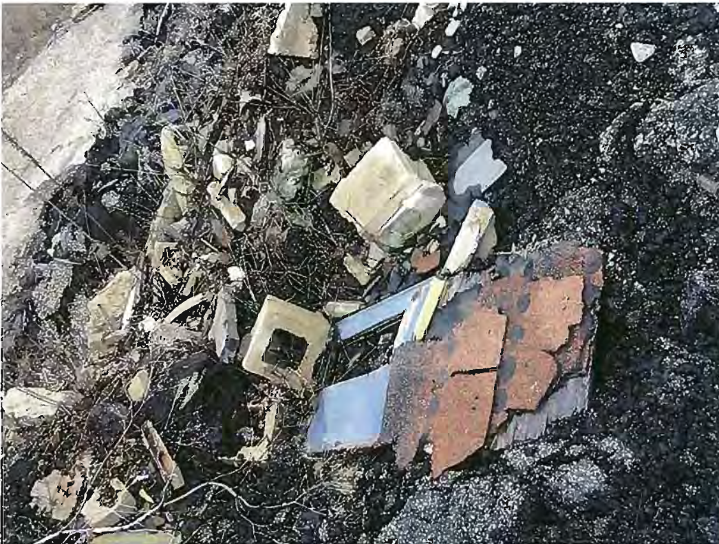
Date:02-10-2012 Time: 11:23AM Direction: Southeast Photo by: Jen O'Hearn Exposure #: 020 Comments: View of shingles, dimensional lumber, demolition debris, concrete block, etc. on top of asphalt pile.
