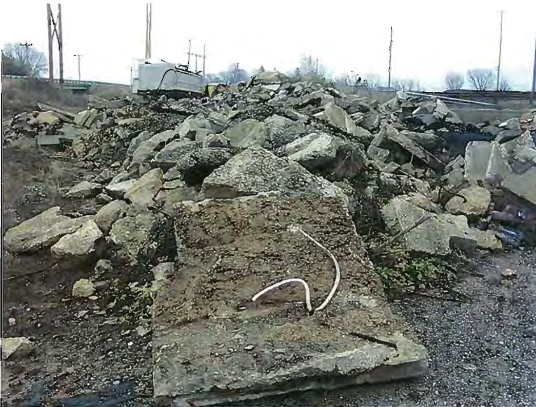
Date:02-10-2012 Time: 11:24AM Direction: East Photo by: Jen O'Hearn Exposure #: 021 Comments: View of conduit with wiring, concrete with protruding rebar, etc.
